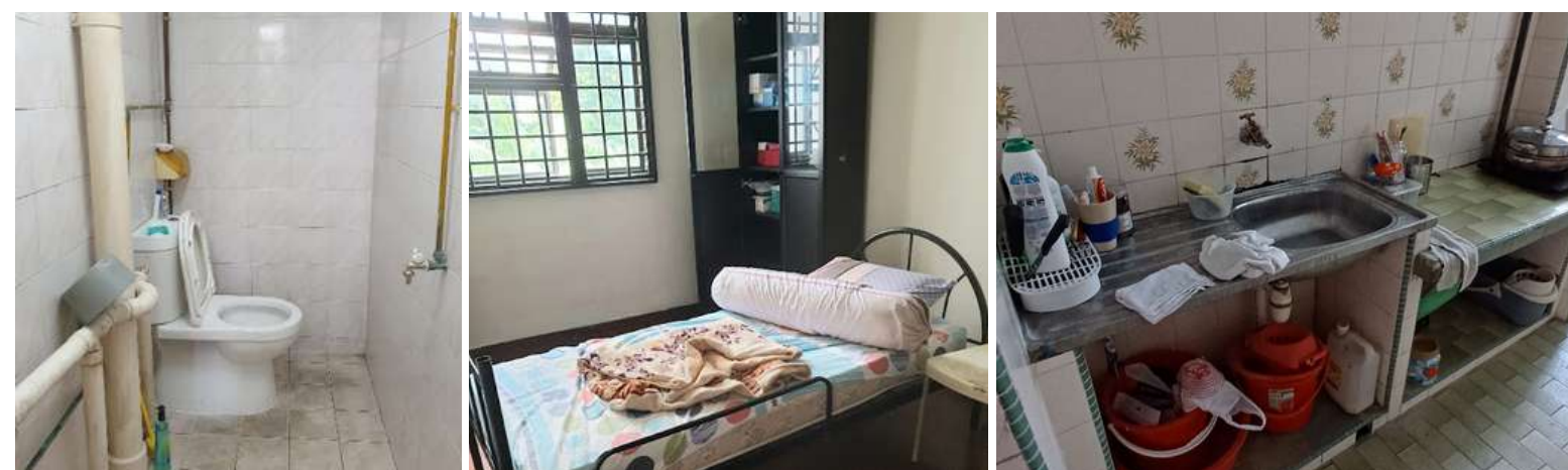
After: Significant changes made for Mr P's home after we cleaned and painted his house
